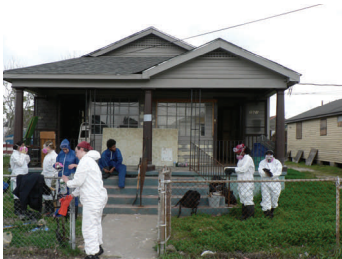
A group of volunteers preparing to gut out a house in the Upper 9th Ward.
